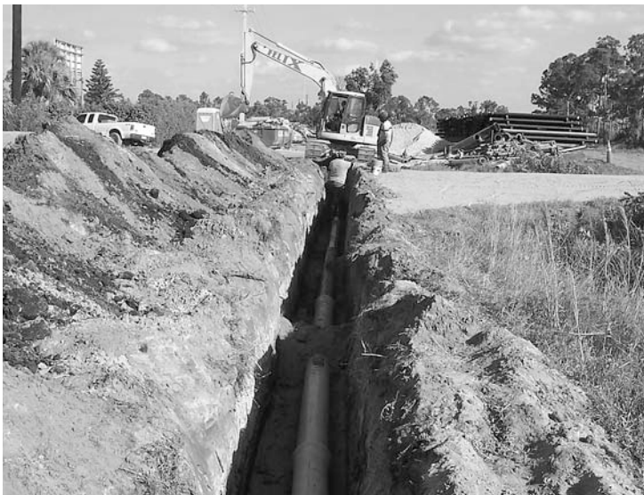
Installation of potable water service in PBCE is on schedule for February 2008 completion
